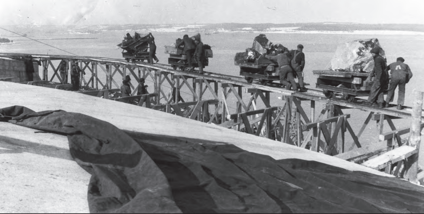
Dumping granite fill on the harbourward face of Connaught Battery from the light rail system that assisted construction. This photo was likely taken in early 1916.
